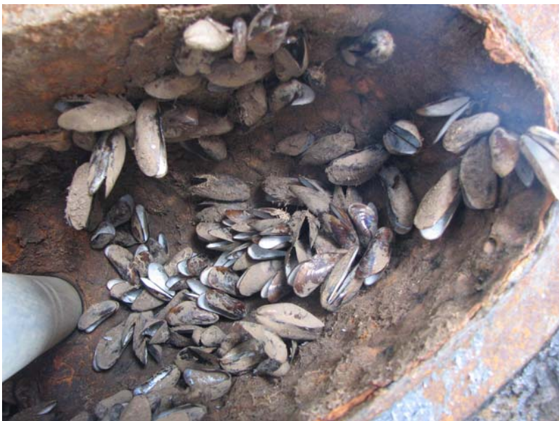
Figure 1. Freshwater exotic asian mussel Limnoperna fortunei (Dunker, 1857) "macrofouling" in Oil Refinery installations, Sinos River Basin region, Canoas Municipal District, Rio Grande do Sul State - RS. Photo : Paulo Lenhard.
