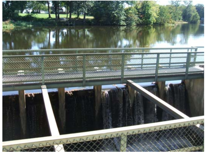
Figure 1. The spillway separating Horseys Pond from Meadow Branch, looking toward the pond
